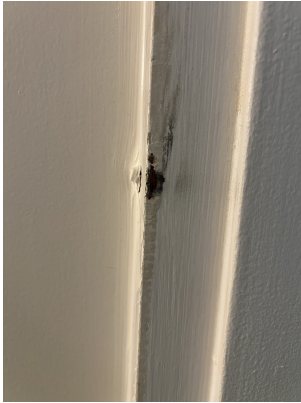
Hazard: Bathroom 1 | Door Casing | Deteriorated Paint
