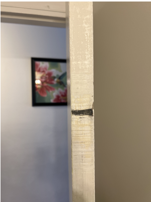
Hazard: Bathroom 2 | Door Casing | Deteriorated Paint
