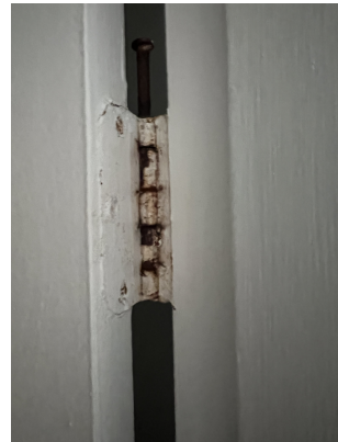
Hazard: Bathroom 2 | Door | Deteriorated Paint
