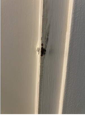
Hazard: Bathroom 1 | Door Casing | Deteriorated Paint
