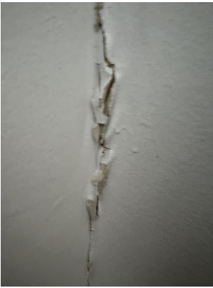
Hazard: Stairwell 1 | Wall | Deteriorated Paint
