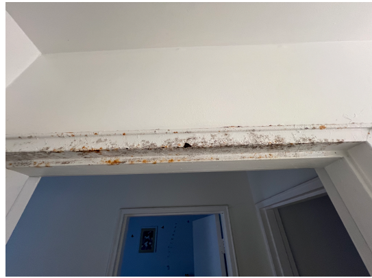
Hazard: Stairwell 1 | Wall | Deteriorated Paint
