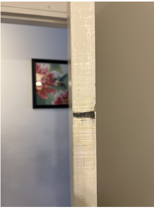
Hazard: Bathroom 2 | Door Casing | Deteriorated Paint
