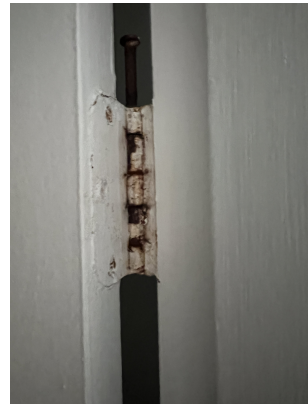
Hazard: Bathroom 2 | Door | Deteriorated Paint
