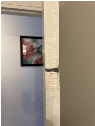
Hazard: Bathroom 2 | Door | Deteriorated Paint
