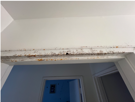
Hazard: Bathroom 2 | Door Casing | Deteriorated Paint
