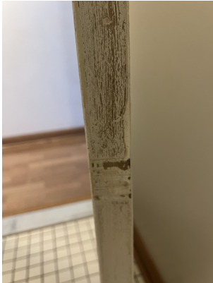
Hazard: Bathroom 1 | Door | Deteriorated Paint
