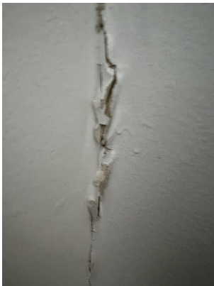
Hazard: Stairwell 1 | Wall | Deteriorated Paint
