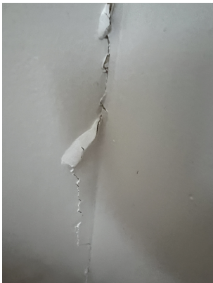
Hazard: Stairwell 1 | Wall | Deteriorated Paint
