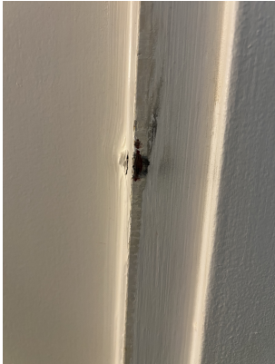
Hazard: Bathroom 1 | Door Casing | Deteriorated Paint
