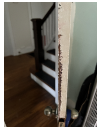
Hazard: Bedroom 1 | Door | Deteriorated Paint
