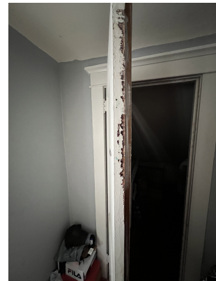
Hazard: Bedroom 3 Closet wall A | Door | Deteriorated Paint
