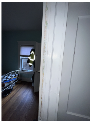
Hazard: bedroom 2 closet | Door Casing | Deteriorated Paint
