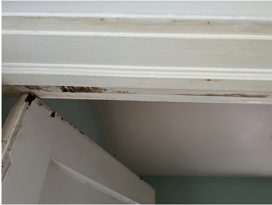
Hazard: Bedroom 1 | Door Casing | Deteriorated Paint
