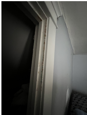
Hazard: Bedroom 3 Closet Wall A | Door Casing | Deteriorated Paint
