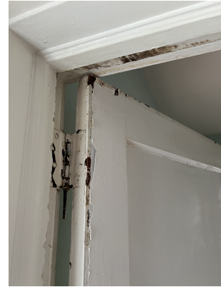
Hazard: Bedroom 1 | Door | Deteriorated Paint
