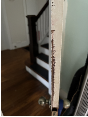
Hazard: Bedroom 1 | Door | Deteriorated Paint
