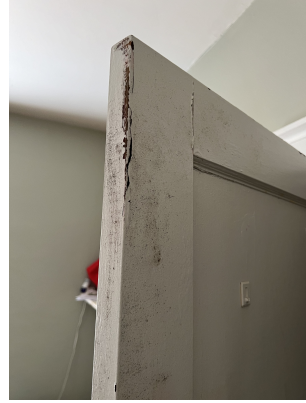
Hazard: Bedroom 1 Closet | Door | Deteriorated Paint
