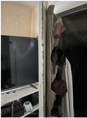
Hazard: Bedroom 3 Closet | Door | Deteriorated Paint
