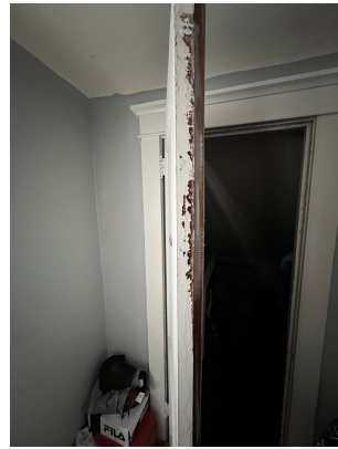
Hazard: Bedroom 4 Closet | Door | Deteriorated Paint
