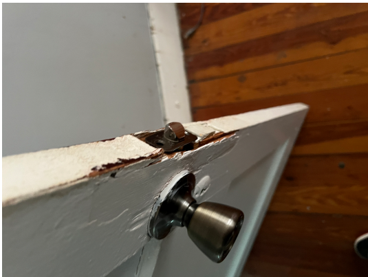
Hazard: Bedroom 5 | Door | Deteriorated Paint
