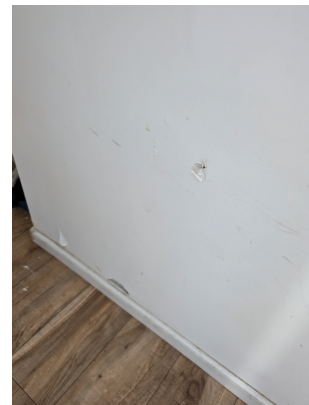
Hazard: Foyer | Wall | Deteriorated Paint
