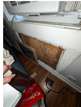
Hazard: Bedroom 5 | Wall underneath Window | Deteriorated Paint
