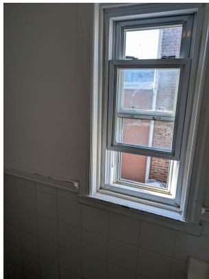
Hazard: Bathroom | Window Casing & Chair Rail Wall Trim | Deteriorated Paint
