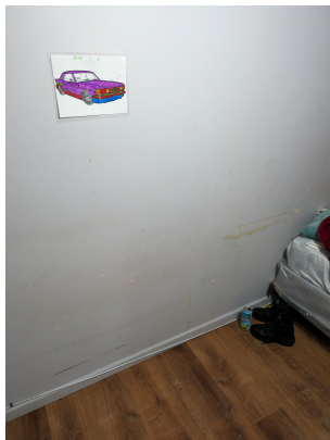
Hazard: Bedroom 3 | Wall | Deteriorated Paint
