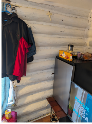
Hazard: Bedroom 1 | Wall | Deteriorated Paint
