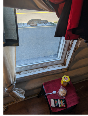
Hazard: Bedroom 1 | Window Casing/Stop | Deteriorated Paint
