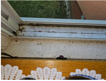
Hazard: All Rooms | All Windows | Dust
