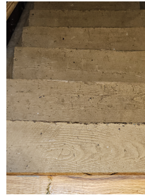
Hazard: Basement Stairwell | Steps | Deteriorated Paint
