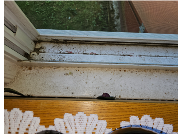
Hazard: All rooms | Baseboard | Dust
