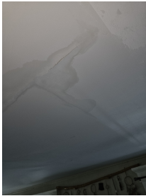
Hazard: Kitchen | Ceiling | Deteriorated Paint
