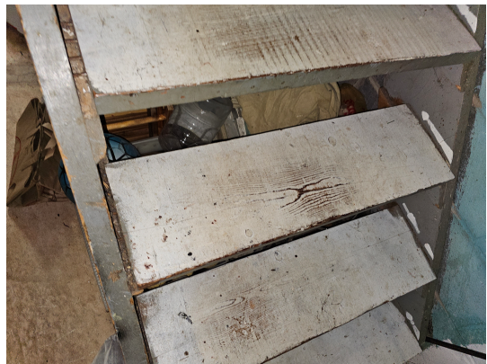
Hazard: Basement | Steps | Dust
