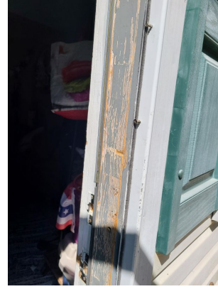
Hazard: Living Room | Closet Door Frame | Deteriorated Paint
