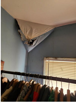
Hazard: Living Room | Wall A and Ceiling | Cracking / Peeling
