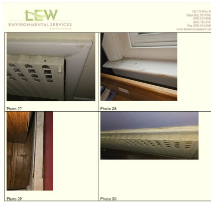
Hazard: Living Room | Baseboard heating cover | Deteriorated Paint
