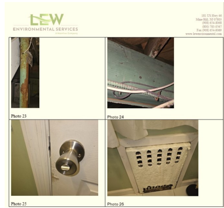
Hazard: Bedroom 2 | radiator | Deteriorated Paint
