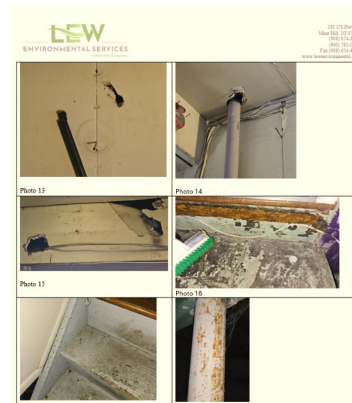
Hazard: Basement | Lolly Column | Deteriorated Paint
