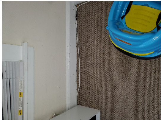
Hazard: Sun Room | Baseboard | Deteriorated Paint
