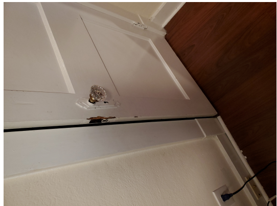
Hazard: Bedroom 3 | Door Casing | Deteriorated Paint
