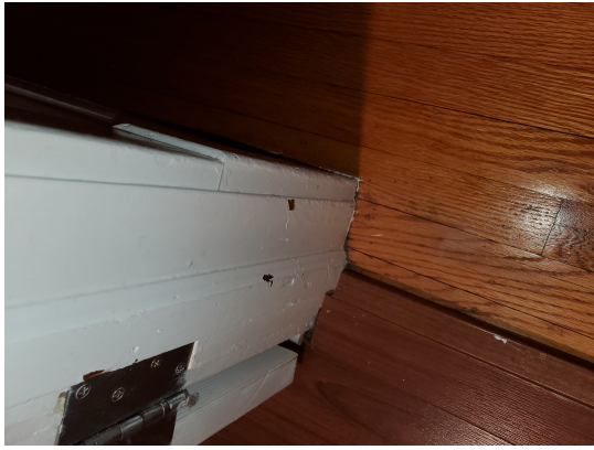
Hazard: Hallway 1 | Door Casing | Deteriorated Paint
