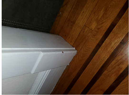
Hazard: Dining Room | Door Casing | Deteriorated Paint
