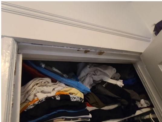
Hazard: Bedroom 3 | Closet Door Jamb and Casing | Deteriorated Paint
