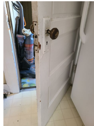
Hazard: Kitchen Door and Casing | Deteriorated Paint
