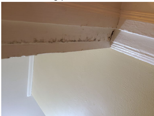
Hazard: Bathroom | Door Jamb | Deteriorated Paint
