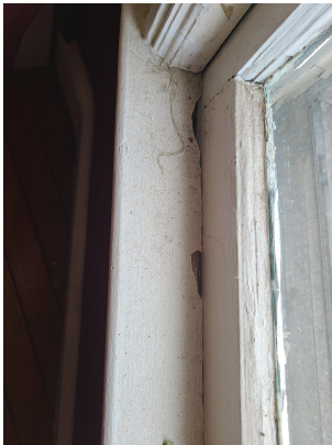
Hazard: Living Room | Window Sill | Deteriorated Paint
