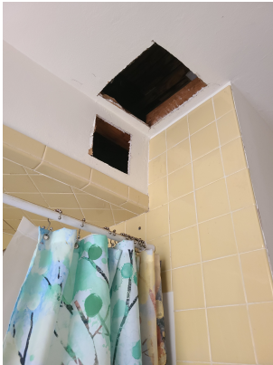
Hazard: Bathroom | Wall and Ceiling | Deteriorated Paint
