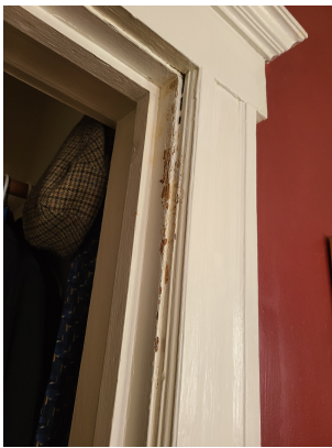
Hazard: Living Room | Closet Door Jamb | Deteriorated Paint
