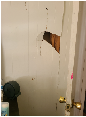
Hazard: Bedroom 2 | Wall C | Deteriorated Paint
