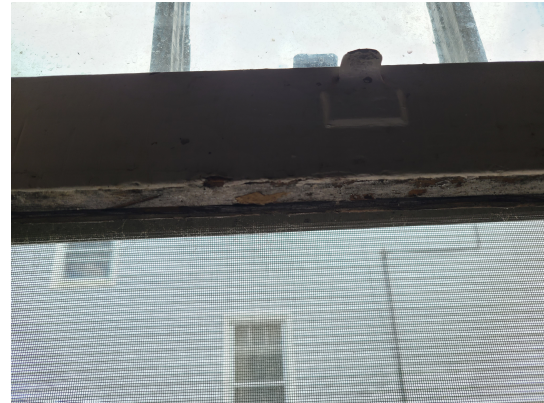
Hazard: Bathroom | Window Sash | Deteriorated Paint
