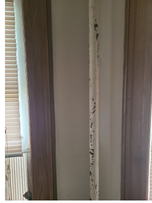
Hazard: Bedroom 1 | Pipe | Deteriorated Paint
