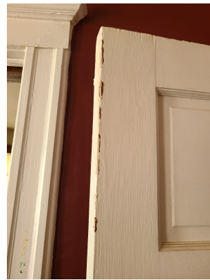
Hazard: Living Room | Door | Deteriorated Paint
