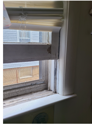
Hazard: Kitchen | Window Sill and Sash | Deteriorated Paint
