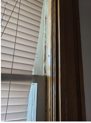
Hazard: Bedroom 1 | Window Sash and Jamb | Deteriorated Paint
