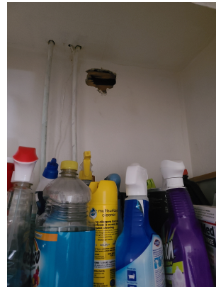
Hazard: Hall | Closet Wall | Deteriorated Paint
