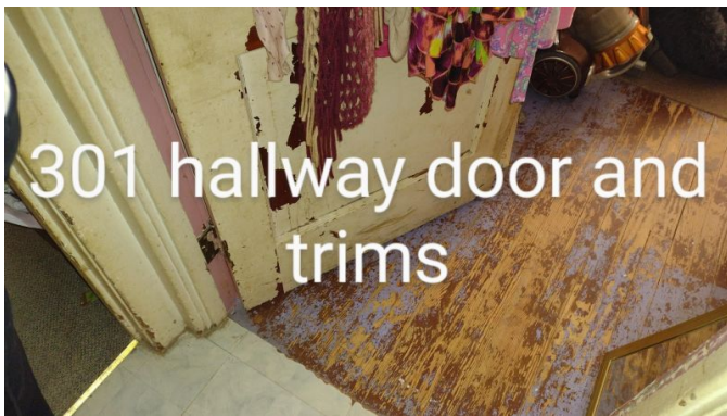
Hazard: Hallway | Door and trims | Deteriorated Paint
