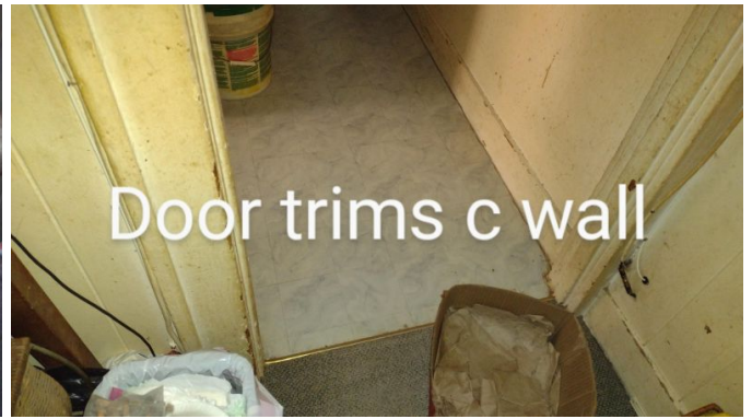
Hazard: Living Room | Door jamb and trims | Deteriorated Paint
