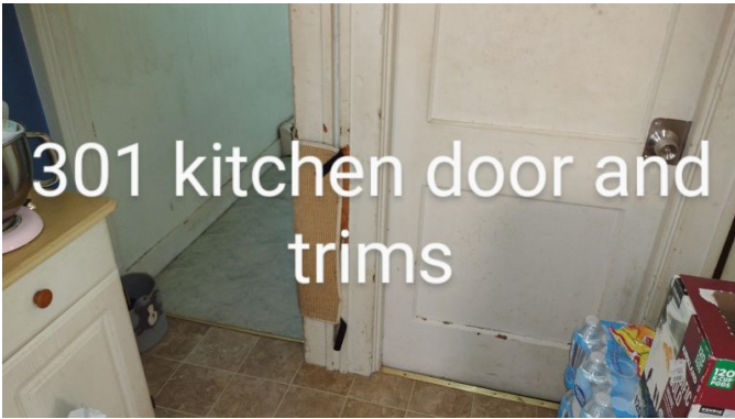
Hazard: Kitchen | Door and trims | Deteriorated Paint
