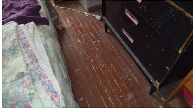
Hazard: Bedrooms 1-2 | Floors | Deteriorated Paint
