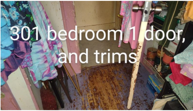
Hazard: Bedroom 1 | Door and trims | Deteriorated Paint
