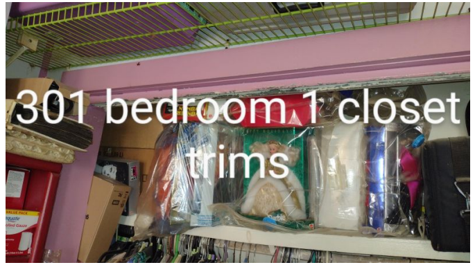
Hazard: Bedroom 1 | Closet door and trims | Deteriorated Paint
