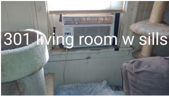
Hazard: Living Room | Window sills | Deteriorated Paint
