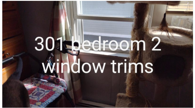
Hazard: Bedroom 2 | Window trims | Deteriorated Paint
