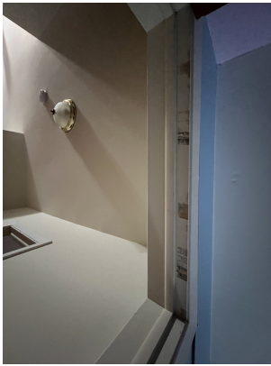
Hazard: Bedroom 2 | Door Casing | Deteriorated Paint
