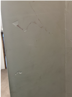
Hazard: Stairwell 1 | Wall | Deteriorated Paint
