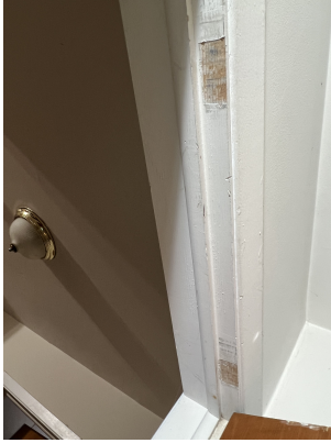
Hazard: Bedroom 1 | Door Casing | Deteriorated Paint
