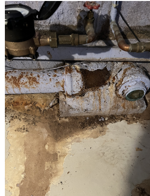
Hazard: Storage Room | Pipe | Deteriorated Paint
