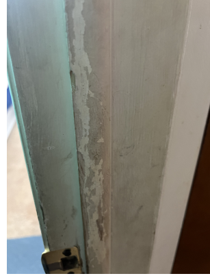
Hazard: Bedroom 1 | Door Casing | Deteriorated Paint
