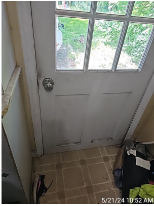
Hazard: Foyer | Door Casing | Deteriorated Paint
