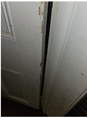
Hazard: Bedroom 2 | Door | Deteriorated Paint
