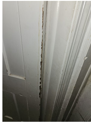
Hazard: Foyer | Baseboard | Deteriorated Paint
