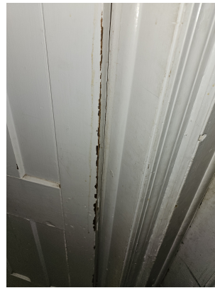
Hazard: Stairwell | Over head trim | Deteriorated Paint
