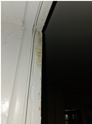
Hazard: Bedroom 2 | Door | Deteriorated Paint
