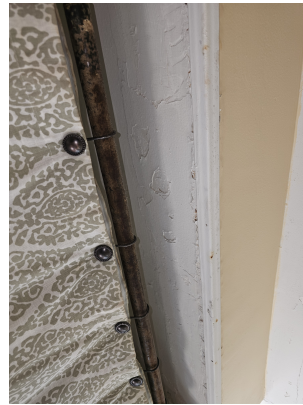
Hazard: Bathroom 1 | Overhead Trim | Deteriorated Paint
