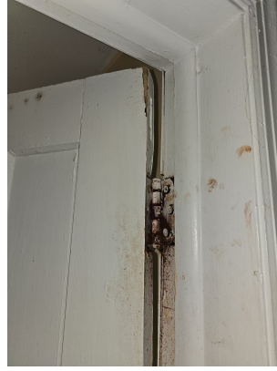
Hazard: Bedroom 1 | Door | Deteriorated Paint
