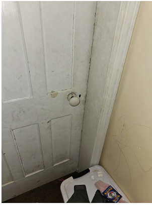
Hazard: Foyer | Door | Deteriorated Paint
