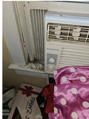
Hazard: Bedroom 2 | Window Sill | Dust
