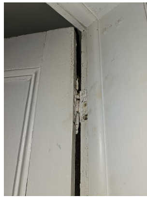
Hazard: Bedroom 2 | Hinge | Deteriorated Paint
