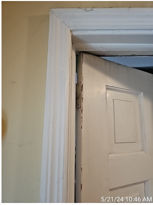
Hazard: Foyer | Door | Deteriorated Paint
