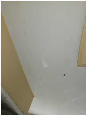
Hazard: Foyer | Ceiling | Deteriorated Paint
