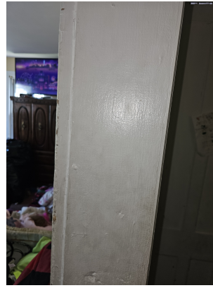
Hazard: Bedroom 2 | Door Jamb | Deteriorated Paint
