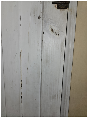
Hazard: Foyer | Door | Deteriorated Paint
