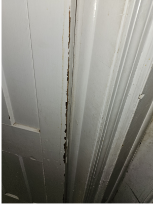
Hazard: Bedroom 1 | Door | Deteriorated Paint
