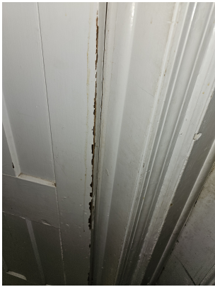
Hazard: Stairwell | Stringer | Deteriorated Paint
