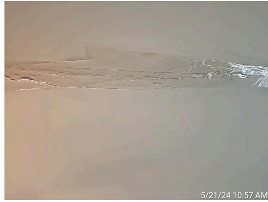
Hazard: Living Room | Ceiling | Deteriorated Paint
