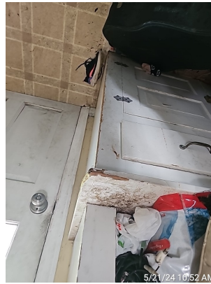
Hazard: Butler's Pantry | Built in Cabinet and Counter | Deteriorated Paint
