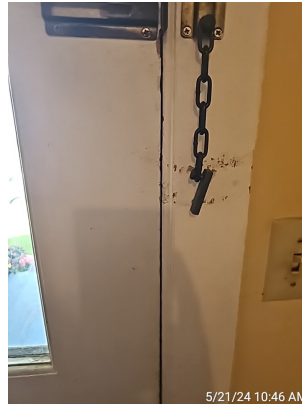
Hazard: Foyer | Door Casing | Deteriorated Paint
