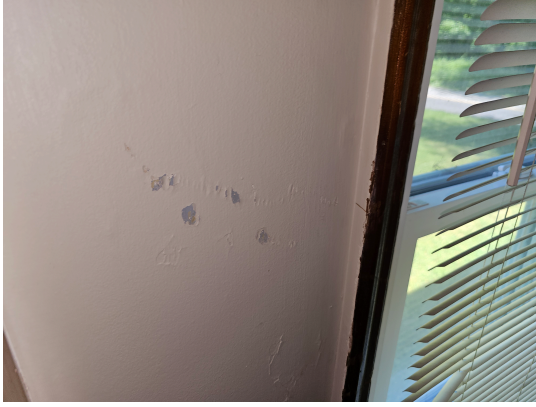
Hazard: Living Room | Wall | Deteriorated Paint
