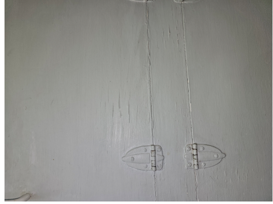
Hazard: Kitchen | upper cabinets | Deteriorated Paint
