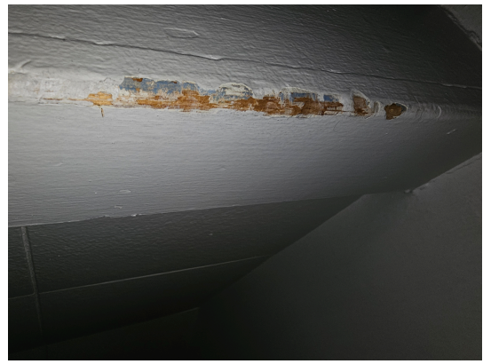
Hazard: Foyer | Baseboard | Deteriorated Paint
