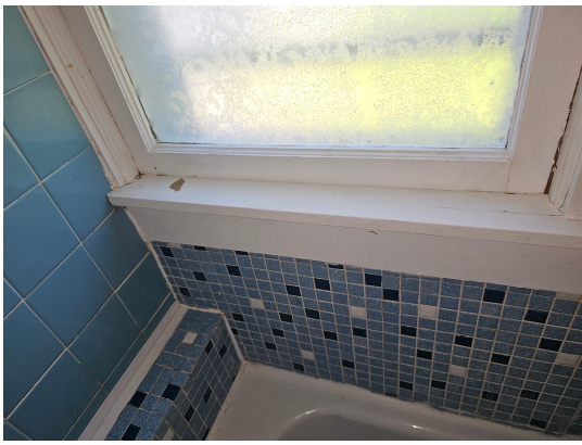
Hazard: Bathroom 1 | Window Sill | Deteriorated Paint
