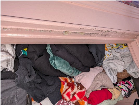
Hazard: Bedroom 1 | Closet Door and Jamb | Deteriorated Paint
