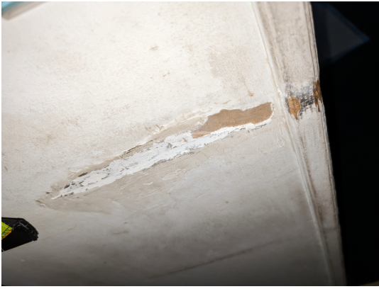
Hazard: Kitchen | Wall | Deteriorated Paint
