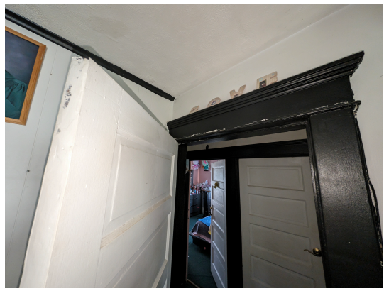
Hazard: Living Room | Door Header | Deteriorated Paint
