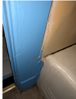
Hazard: Bathroom | Door Casing | Deteriorated Paint
