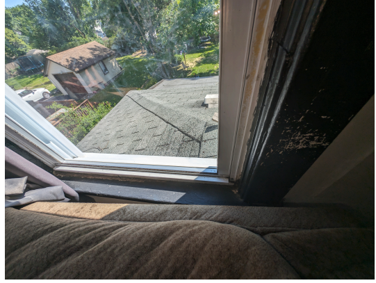
Hazard: Livingroom | Window Sill and Casing | Deteriorated Paint
