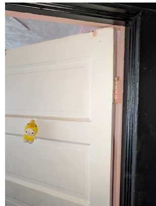
Hazard: Bedroom 1 | Door from foyer | Deteriorated Paint
