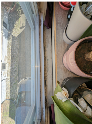
Hazard: Bedroom 2 | Window Sills | Deteriorated Paint
