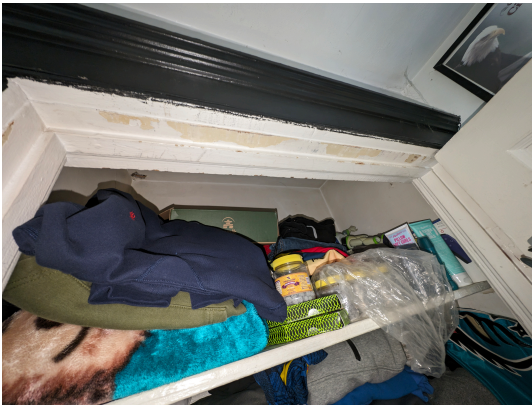
Hazard: Living Room | Closet Door Jamb and Ceiling | Deteriorated Paint
