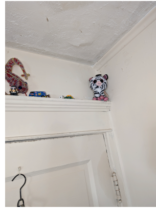
Hazard: Bedroom 2 | Ceiling | Deteriorated Paint
