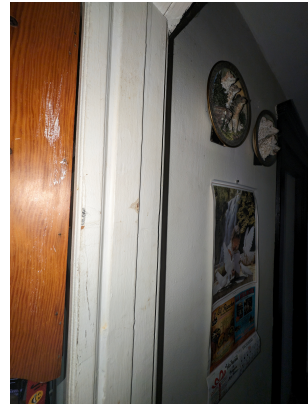
Hazard: Kitchen | Door Casing/Stop | Deteriorated Paint
