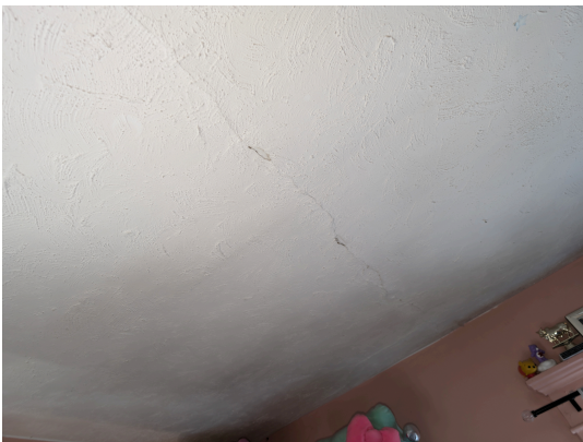
Hazard: Bedroom 1 | Ceiling | Deteriorated Paint
