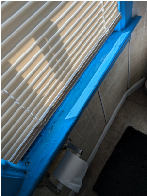
Hazard: Bathroom | Window Sill | Deteriorated Paint
