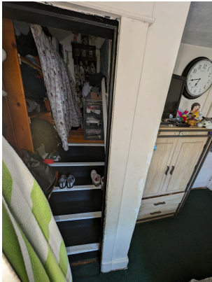
Hazard: Bedroom 2 | Closet Door Casing and Wall | Deteriorated Paint
