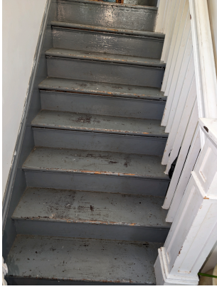
Hazard: Common Hallway | Stair Components | Deteriorated Paint
