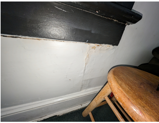
Hazard: Living Room | Wall | Deteriorated Paint
