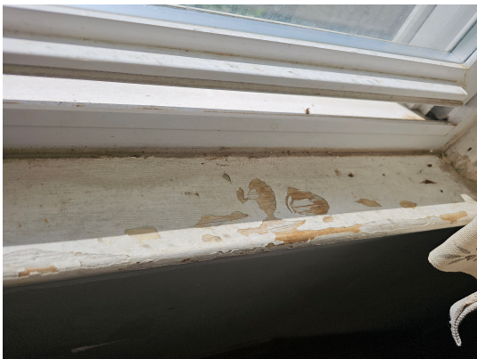
Hazard: Foyer | Window Sill | Deteriorated Paint
