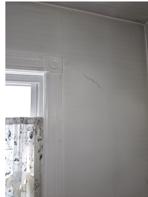
Hazard: Foyer | Door | Deteriorated Paint
