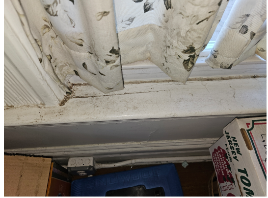
Hazard: Kitchen | Window Sill | Dust
