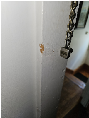
Hazard: Foyer | Baseboard | Deteriorated Paint
