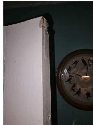
Hazard: Foyer | Door | Deteriorated Paint
