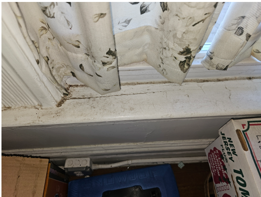
Hazard: Kitchen | Window Sill | Deteriorated Paint
