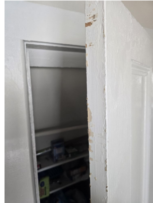
Hazard: Foyer/Hall | Closet Door Components | Deteriorated Paint
