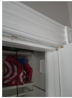
Hazard: Living Room | Closet Door Components | Deteriorated Paint
