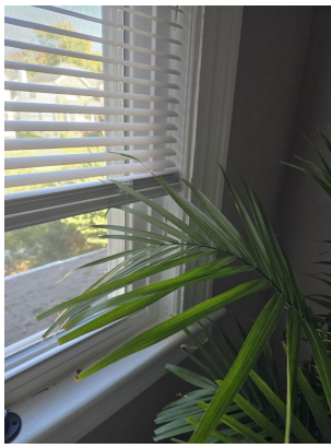
Hazard: Living Room | Window Components | Deteriorated Paint
