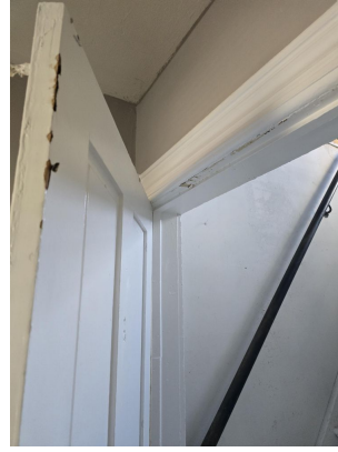
Hazard: Attic Stairwell | Door Components | Deteriorated Paint
