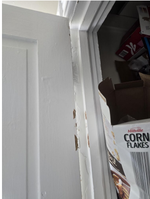
Hazard: Kitchen | Closet Door Components | Deteriorated Paint
