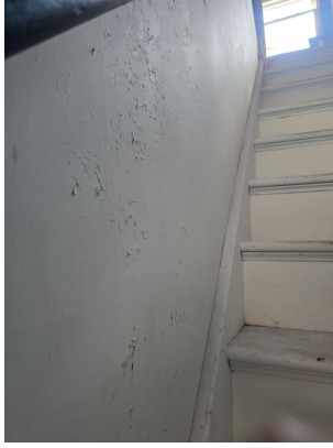
Hazard: Attic Stairwell | Wall | Deteriorated Paint
