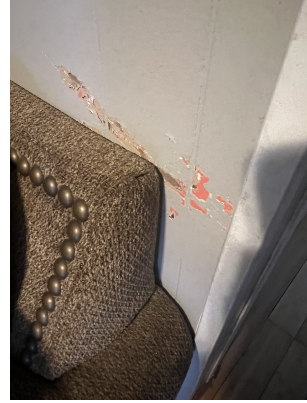
Hazard: Living Room | Wall | Deteriorated Paint
