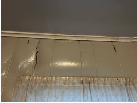
Hazard: Living Room | Wall | Deteriorated Paint
