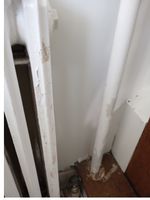
Hazard: Stairhall | pipe and radiator | Deteriorated Paint
