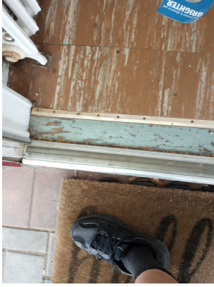
Hazard: Stairhall | Threshold | Deteriorated Paint
