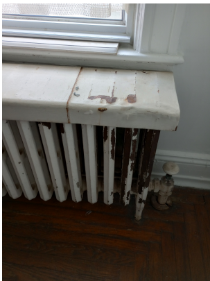
Hazard: Living Room | Radiator | Deteriorated Paint
