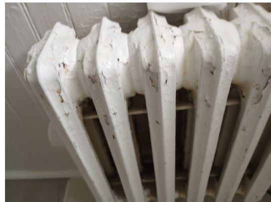
Hazard: Bathroom | Radiator | Deteriorated Paint
