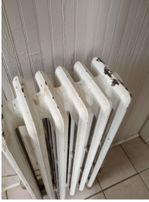
Hazard: Bath | Radiator | Deteriorated Paint
