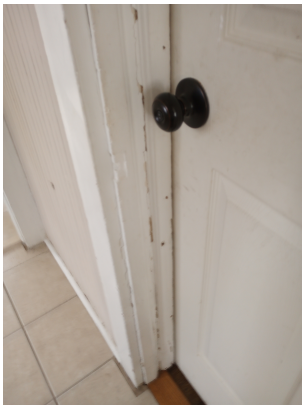
Hazard: Hallway | Door Jamb and Casing | Deteriorated Paint
