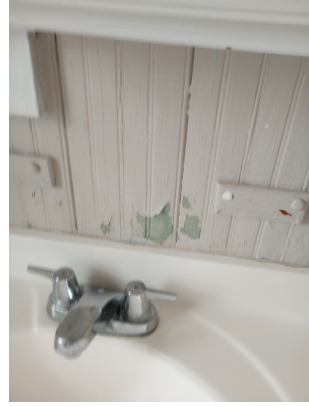
Hazard: Bath | Wall | Deteriorated Paint
