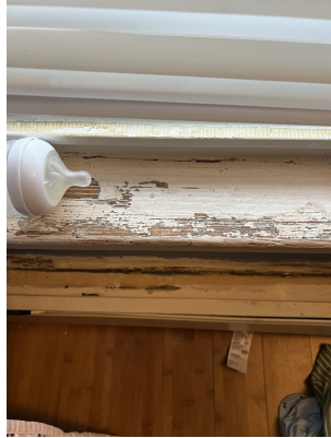
Hazard: Bedroom 2 | Window Sill | Deteriorated Paint
