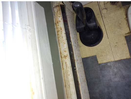
Hazard: Bedroom 1 | Door | Deteriorated Paint
