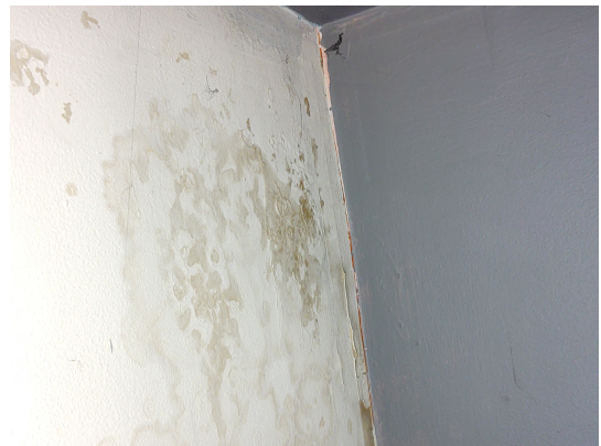
Hazard: Bedroom 2 | Ceiling | Deteriorated Paint
