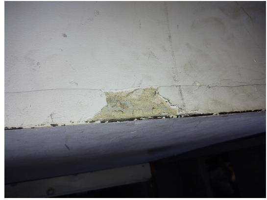
Hazard: Basement | Wall | Deteriorated Paint
