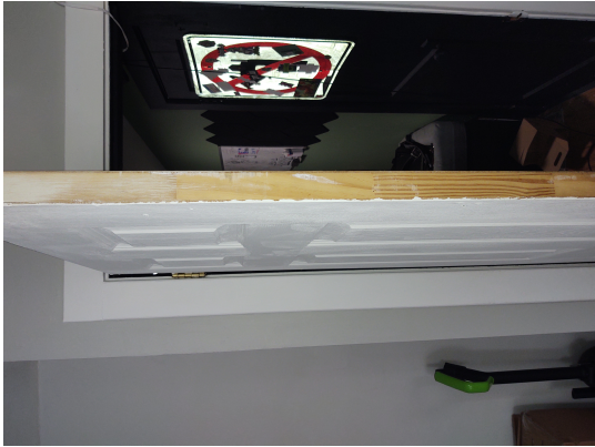
Hazard: Living Room | Door | Deteriorated Paint
