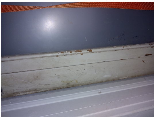
Hazard: Kitchen | Door | Deteriorated Paint
