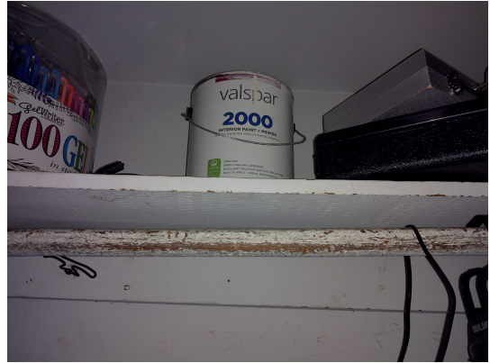
Hazard: Office | Closet Shelf and Clothes Pole | Deteriorated Paint
