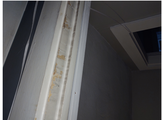
Hazard: Bedroom 2 | Door Jamb | Deteriorated Paint
