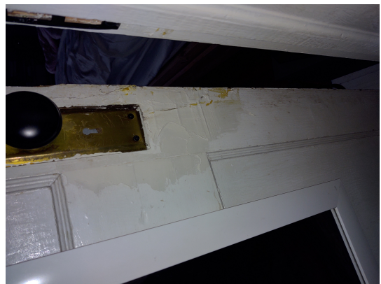
Hazard: Kitchen | Door | Deteriorated Paint
