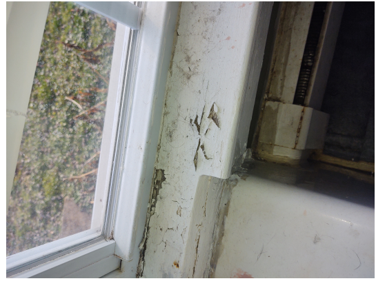
Hazard: Bathroom 1 | Window Sill | Deteriorated Paint
