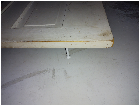
Hazard: Basement | Door | Deteriorated Paint
