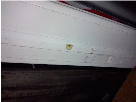
Hazard: Living Room | Door Stop | Deteriorated Paint
