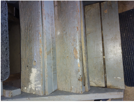
Hazard: Basement | Stair Tread | Deteriorated Paint
