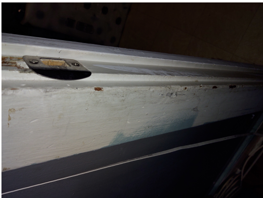
Hazard: Bedroom 2 | Door Casing | Deteriorated Paint
