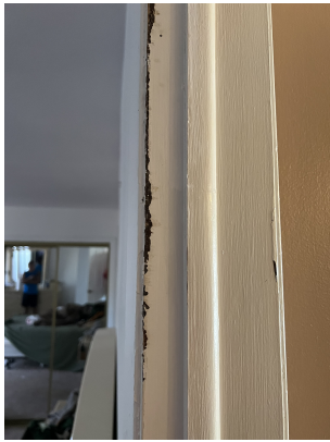
Hazard: Bedroom 1 | Door Casing | Deteriorated Paint
