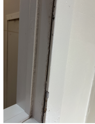
Hazard: Bathroom 3 | Door Casing | Deteriorated Paint
