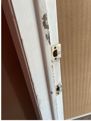
Hazard: Bedroom 2 | Door Casing | Deteriorated Paint
