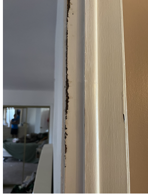
Hazard: Bedroom 1 | Door Casing | Deteriorated Paint
