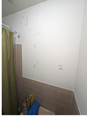
Hazard: Bathroom 1 | Wall | Deteriorated Paint
